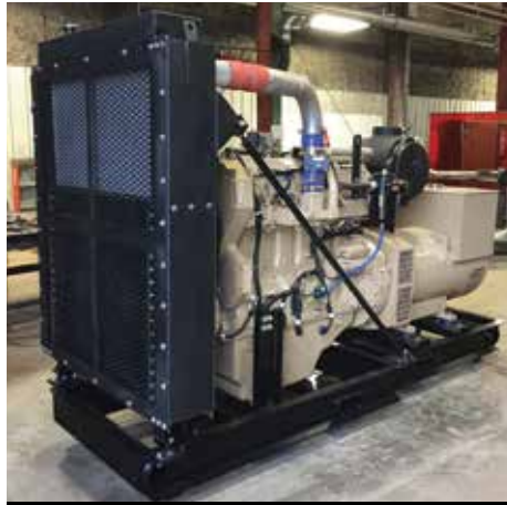
Frontier Power Products in Edmonton designed and built a custom generator that fit the space constraints of the Electric Cuttings Dryer.
